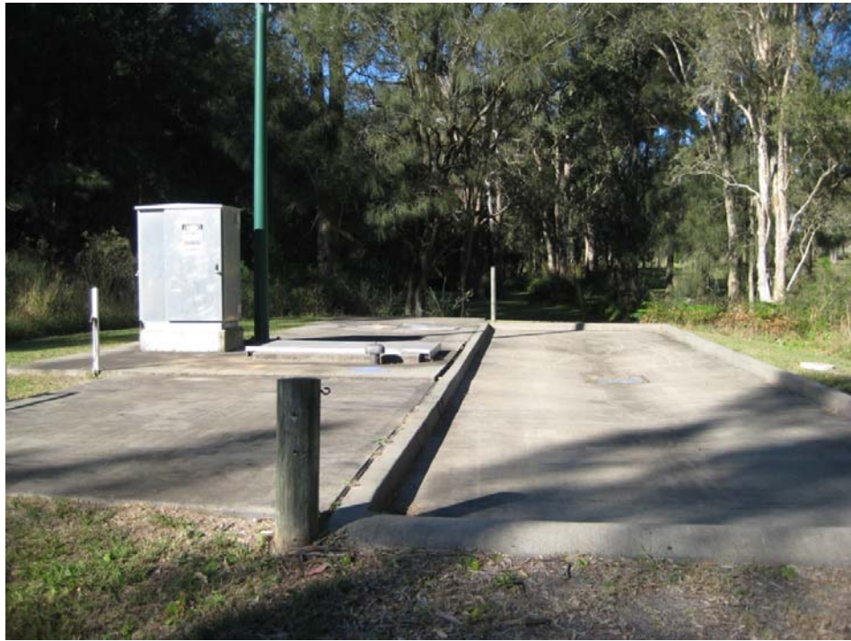
PHOTOGRAPH 9: The Medowie Wastewater Pumping Station, located along the northern boundary of the site
