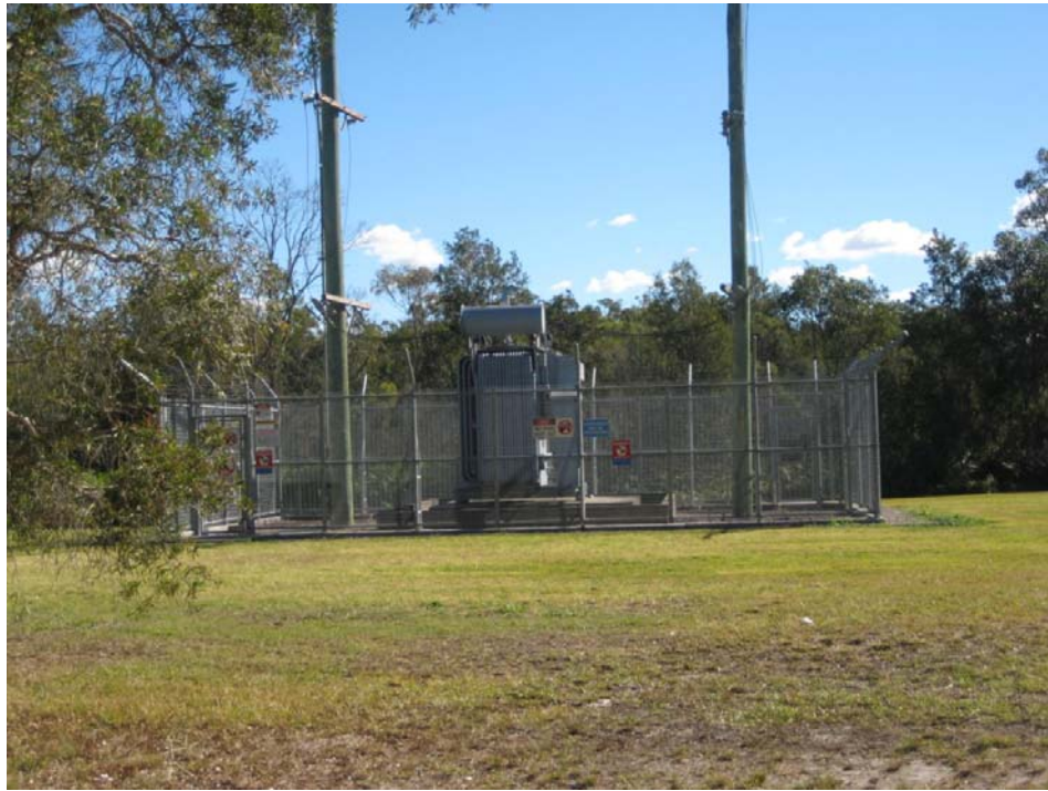
PHOTOGRAPH 1: The electrical substation (transformer yard) located near the middle of the site
