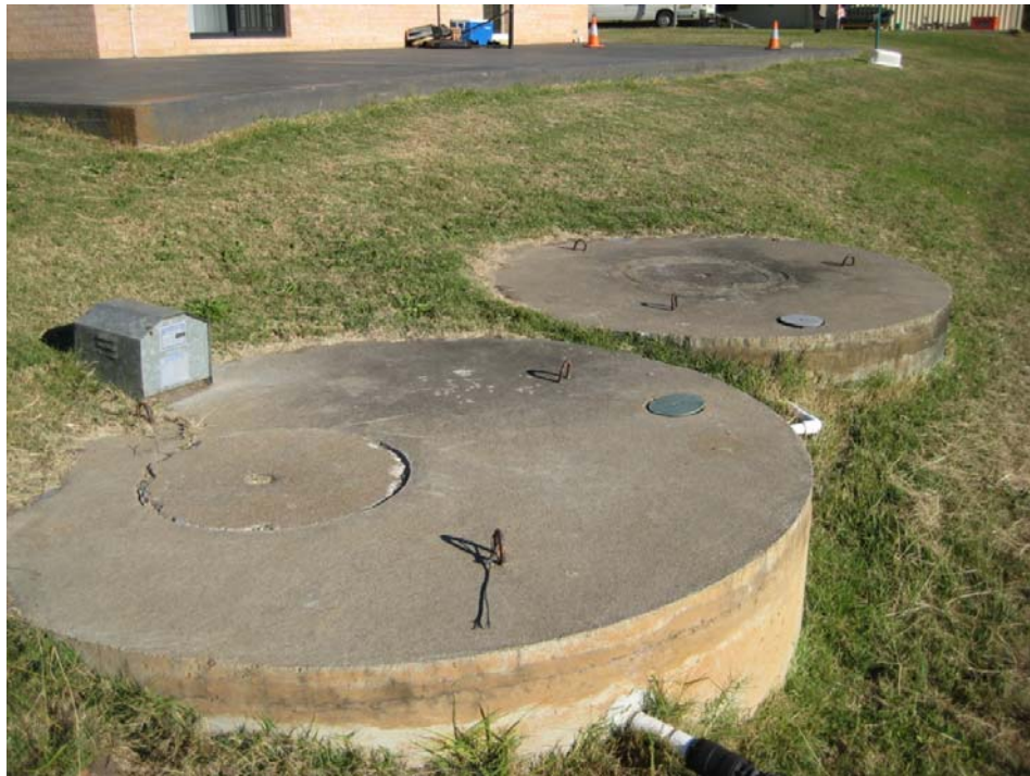
PHOTOGRAPH 12: Septic tanks located near the southernmost house
